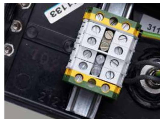
Ex e junction box
